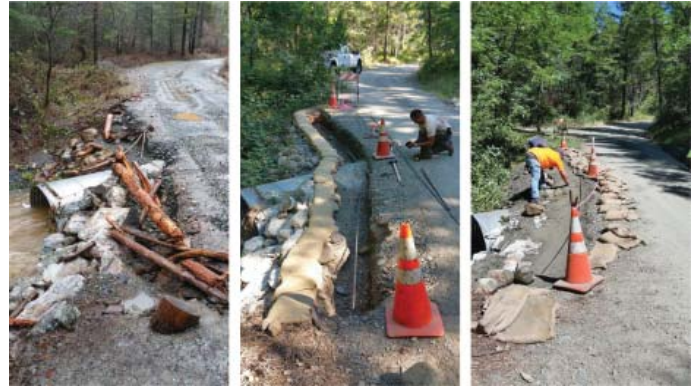
Left to right: After January 2016 overtopping event and the eventual repair in June 2016.
