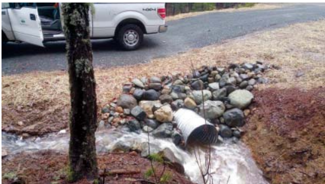
South Roundy Road under high flows in February 2017.
