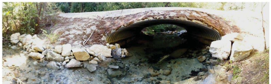
Before, during and after abutment repair on bottomless arch culvert from Upper Grass Valley Creek, view downstream.
