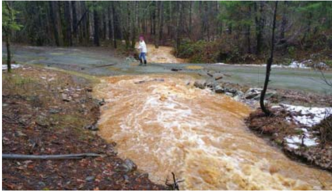
January 20th, 2016: China Gulch overtopped the roadway twice, causing damage to the outboard edge of Blue Rock Road as shown to the right.
