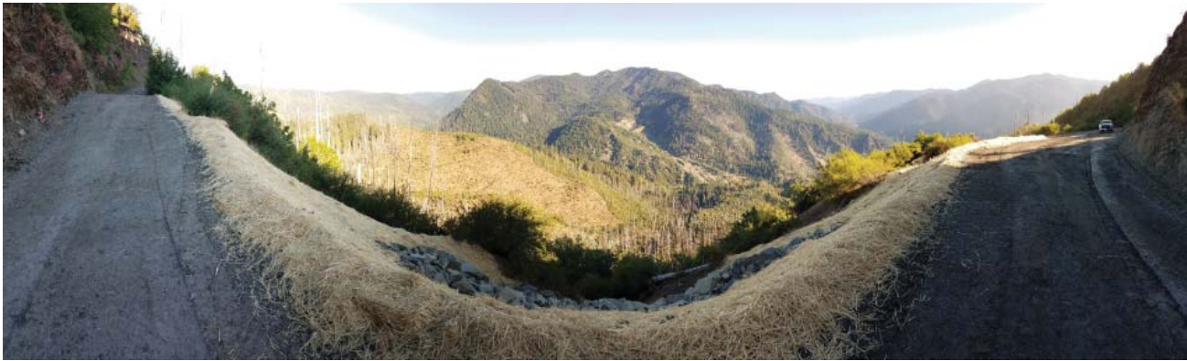
Sims Fire landslide stabilizing on 4N31 in Grouse Creek Watershed, South Fork Trinity Rver.
