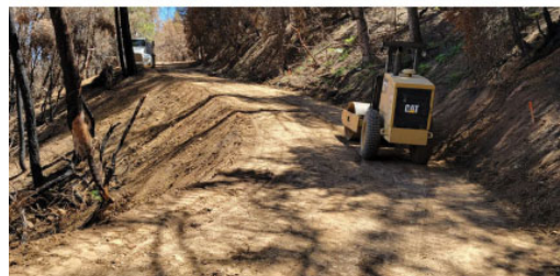
A repaired hole in the road created by a burned-out stump
