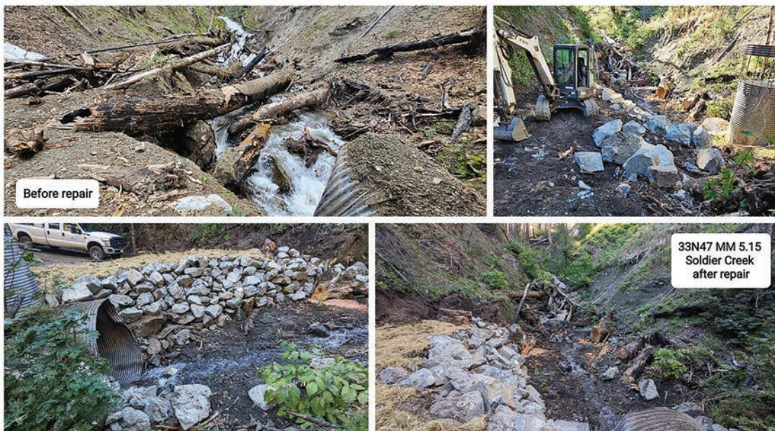
Large log jam was cleared from inlet basin of tributary to Soldier Creek in the Monument Fire area and rip rap was installed to eliminate bank erosion.
