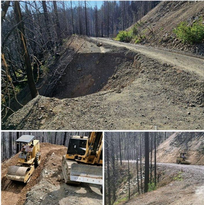
Fill failure repair on Wild-Mad Road (30 Road) in Upper Bierce Creek, Shasta -Trinity National Forest.
