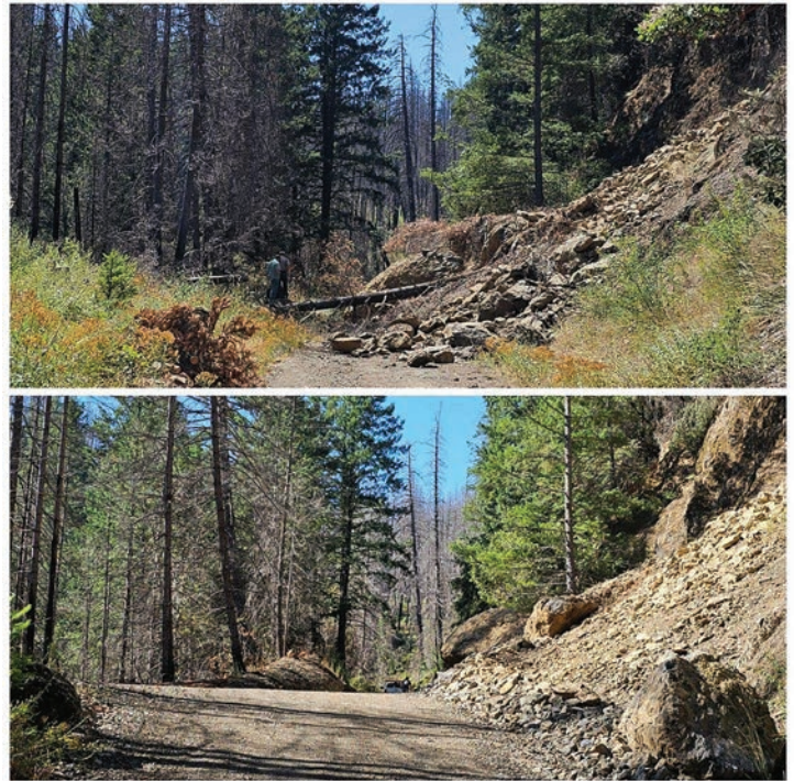
Rock slide cleared from road along Ruth Lake, Six Rivers National Forest , 1S06 Road
