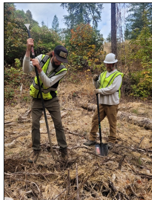
Tyler McKinley and Tim Asgeirsson digging the first hole at the Hayfork Culverts II revegetation site.
